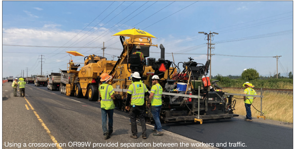
Using a crossover on OR99W provided separation between the workers and traffic.
